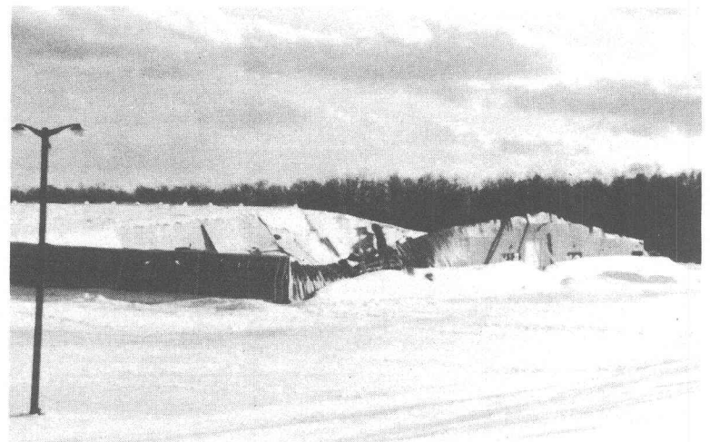
ROOF CAVES — The Feast building at Mount Pocono, Pa., suffered a disastrous cave-in Jan. 28 after snow and ice accumulated on its roof during a storm. The damage may mean no Feast at the Poconos in 1978. (See article, page 1.)
