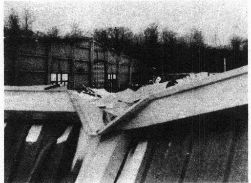
DISASTER — The roof of the Church-owned Festival building at Mount Pocono, Pa., collapsed under the weight of snow during a blizzard Jan. 28.
